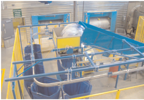
FLM'S FULLY AUTOMATED LOADING SYSTEM
